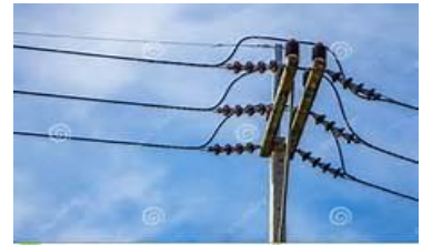
Skywire is nearby zero voltage connected to earth (Fig -2)
