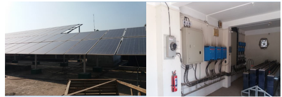
Solar Charging Station at Chandra, Gazipur. Under Dhaka PBS-1
