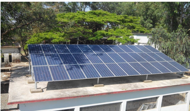
Solar Power Plant at Teknaf Upazila Complex
