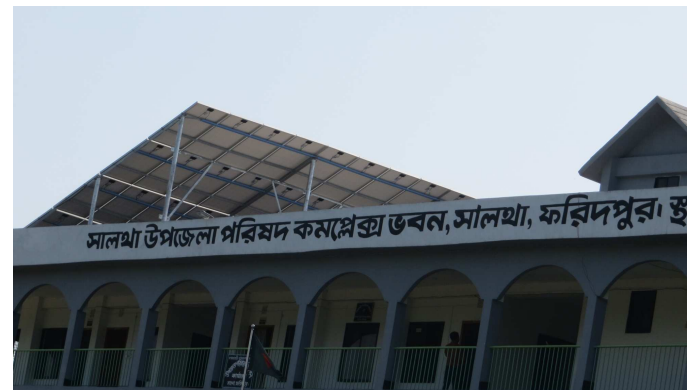
Solar Power Plant at Saltha Upazila Complex
