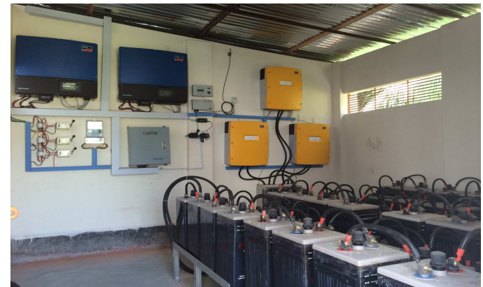
Battery & Inverter Room
