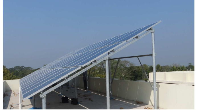
Solar Power Plant at Tungipara Upazila Complex
