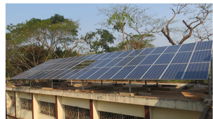
Solar Power Plant at Rajoir Upazila Complex
