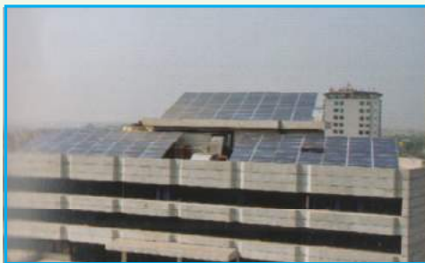
49 kWp BREB Rooftop Solar Power Plant
