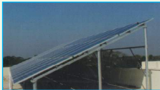
30 kWp Solar Power Plant at Tungipara Upazila Complex
