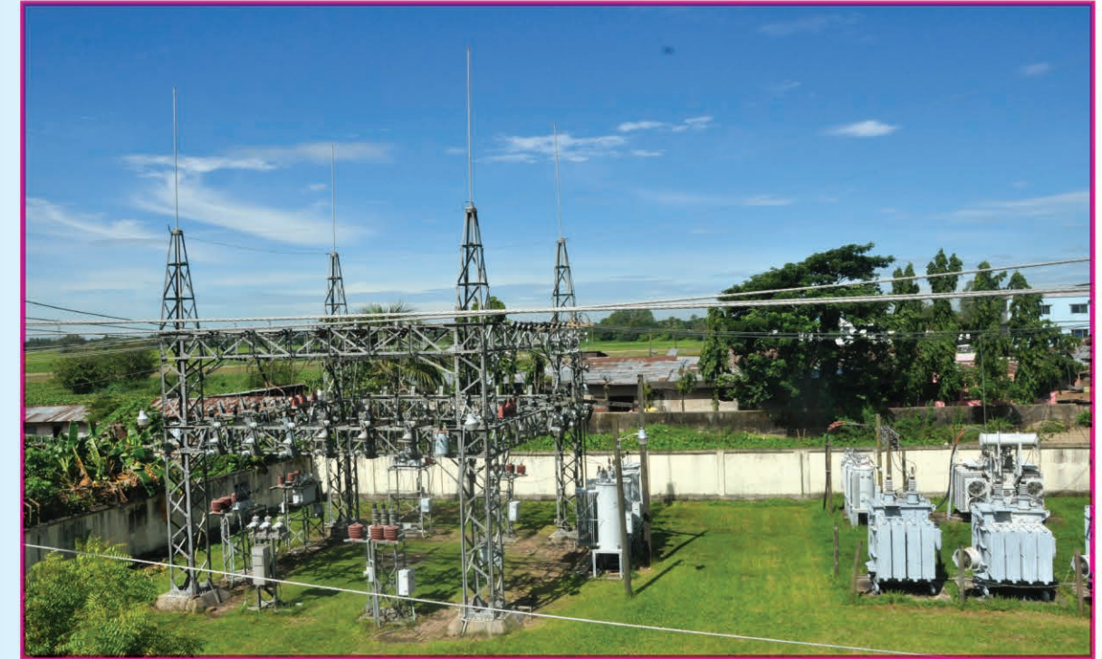
Distribution sub-station of Bangladesh Rural Electrification Board
